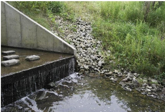
Photograph 3: Outlet of crossing structure at Coleraine Drive; looking at left bank on August 10, 2017
